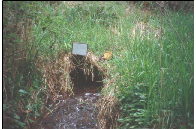
Figure 77. 993724 Before Construction: The old crossing was a round corrugated steel culvert with a 4.3 ft diameter, measuring 204 ft long. The crossing was a barrier due to the slope.
