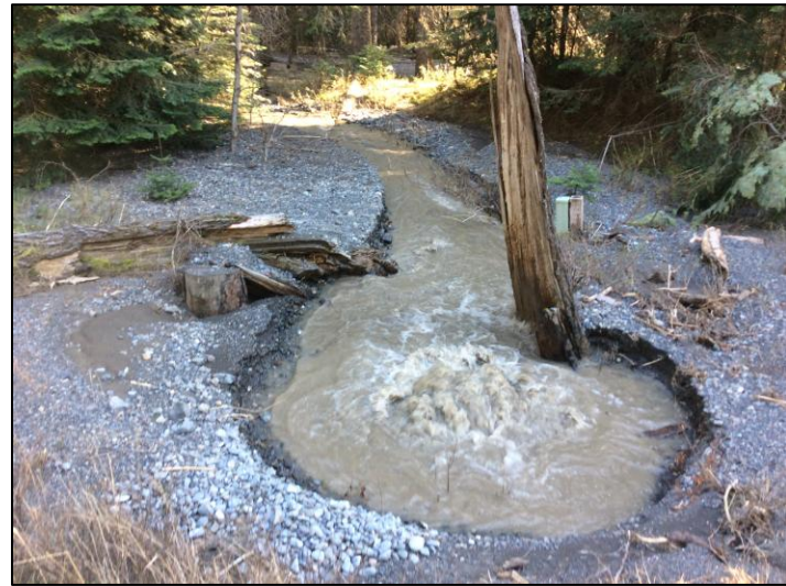
Figure 88. 998490 Before Construction: Outlet during a high flow event in 2016. The culvert was plugged with sediment and required an emergency cleaning.
