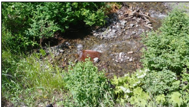
Figure 87. 998490 Before Construction: Inlet in June 2018. The old crossing was a 3 ft diameter, 55 ft long, corrugated metal culvert that was almost completely filled with sediment and debris. The outlet was buried below the channel bed.
