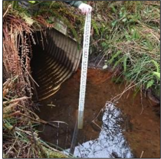
Figure 67. 997363 Before Construction: The old crossing was a 4 ft diameter corrugated steel culvert and was a barrier due to slope.
