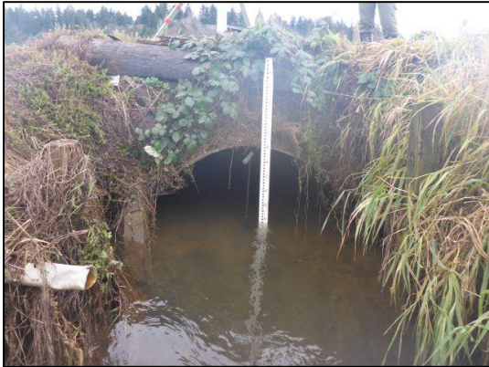
Figure 24. 935158 Before Construction: This crossing was a single corrugated steel squashed culvert with a span of 5.5 ft and a rise of 4 ft. The culvert length was 66.5 ft long and provided access to a large agricultural area. During the previous site assessment, it was determined that this site was not a barrier to fish passage.
