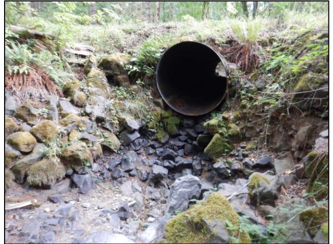
Figure 33. 991672 Before Construction: The former structure was a 5 ft diameter corrugated steel culvert that ran a length of 53 ft underneath SR 108. A water surface drop of 1.5 ft at the outlet created barrier conditions that limited upstream migration.
