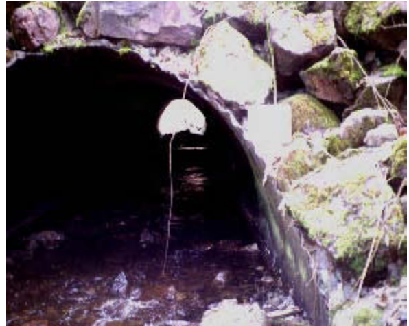
Figure 27. A 3 m wide structural plate steel arch culvert was equipped with steel baffles. The small baffles were not effective at improving passability throughout the 4% slope culvert.
