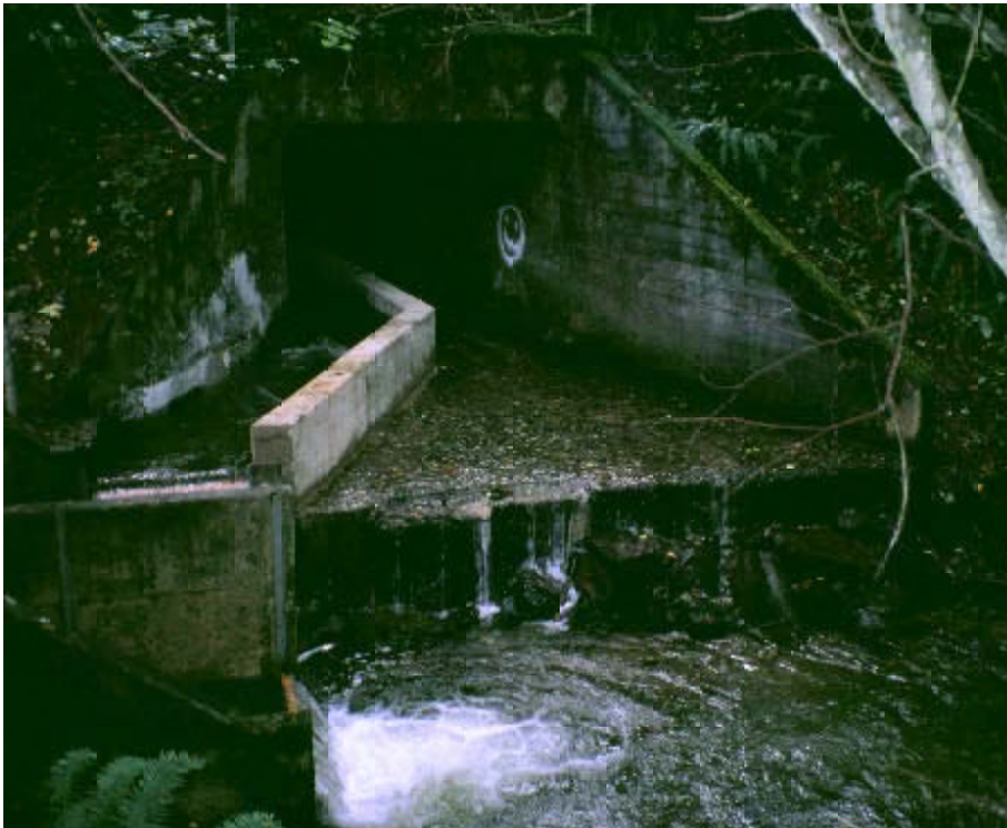
Figure 16. A single, 3 m wide concrete box culvert equipped with fifty-three sets of baffles and a four step weir-pool fishway downstream of the culvert provided fish passage only at a narrow range of flows. Accumulated debris and sediments must be removed from the fishway on an annual basis. In 2004 WSDOT contracted with WDFW to provide improvements to the Ennis Creek fishway. Improvements included raising the center wall of the fishway, removal of a few baffles, and rearranging
