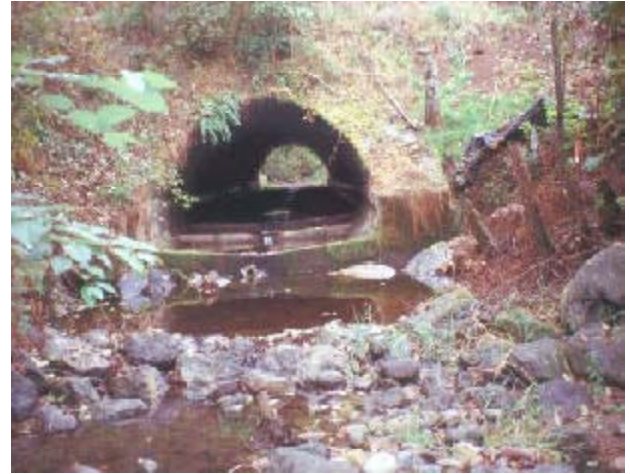
Figure 10. A structural steel plate arch culvert, 4.6 m wide, equipped with 13 concrete weirs and three rock controls downstream of the culvert was identified as a barrier due to excessive hydraulic drop of 0.48 m at one of the weirs.
