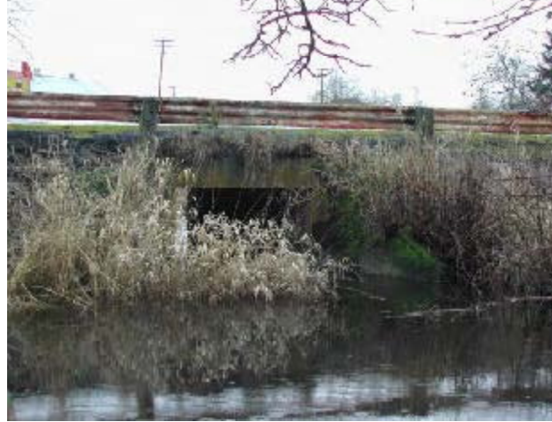
Figure 24. The original precast concrete, 1.52 m wide single box culvert was undersized.
