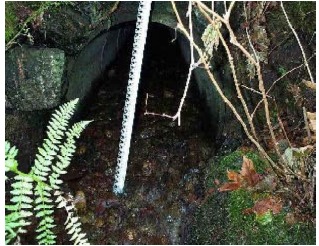
Figure 21. A round, 0.76 m wide concrete culvert was undersized.
