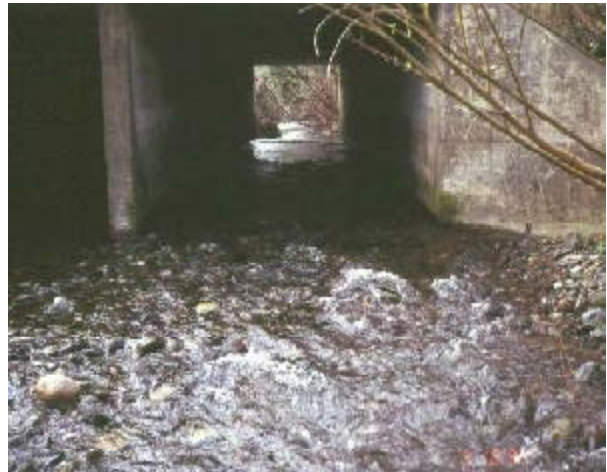
Figure 13. A 2.44 m wide concrete double box culvert, equipped with steel baffles was not providing adequate fish passage due to an excessive water velocity inside the culvert. In addition, the culverts needed frequent maintenance as a result of aggradation and debris accumulation, especially during the threatened summer chum run.
