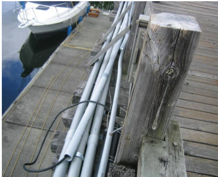
Figure 3.31. Utility lines on a dock in Gig Harbor. Photo: Washington DNR
